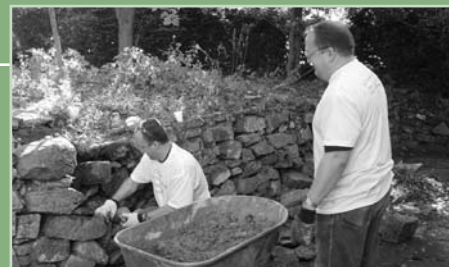
Centocor volunteers rebuilt failing retaining walls along with a myriad of other projects at PRC's Environmental Living Demonstration Center.
